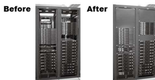
Figure 8: A server rack shown prior to and after the installation of blanking panels. (Photo courtesy of PlenaForm Systems EXIT and EDP Europe EXIT.)
